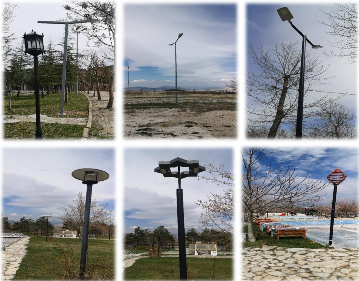
Figure 6. Lighting units in Gökçay promenade
