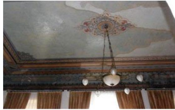
Figure 2. Deterioration in the ceiling due to extinguishing the fire (Source: Istanbul No. 5 Cultural Heritage Preservation Board Regional Directorate Archive)
